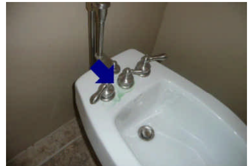
Evidence of past leak
