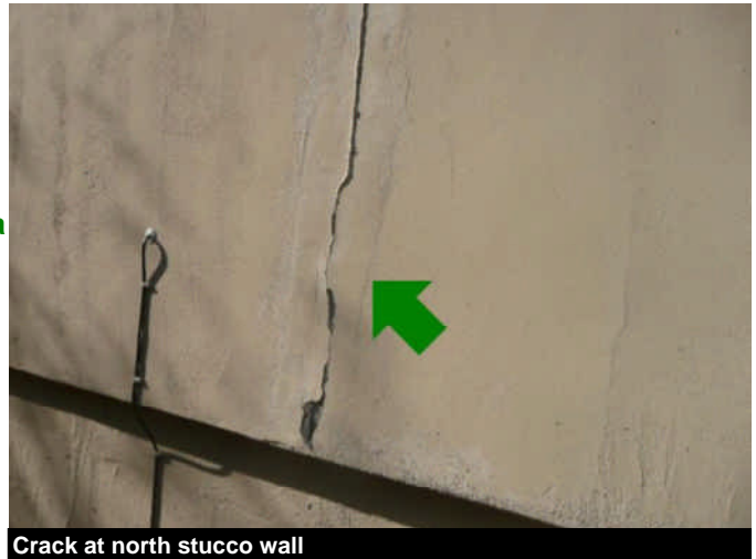
Crack at north stucco wall
