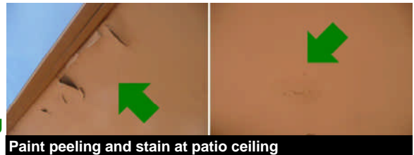
Paint peeling and stain at patio ceiling
