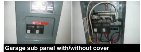
Garage sub panel with/without cover
