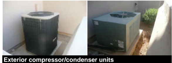
Exterior compressor/condenser units
