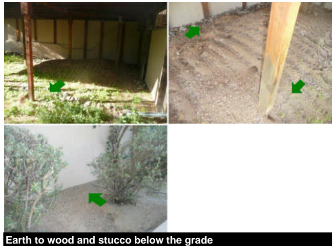
Earth to wood and stucco below the grade
