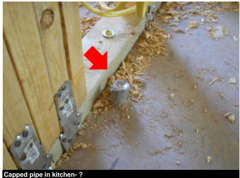
Capped pipe in kitchen- ?
