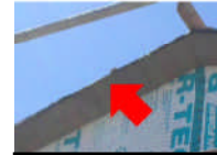
Improper felt installation
