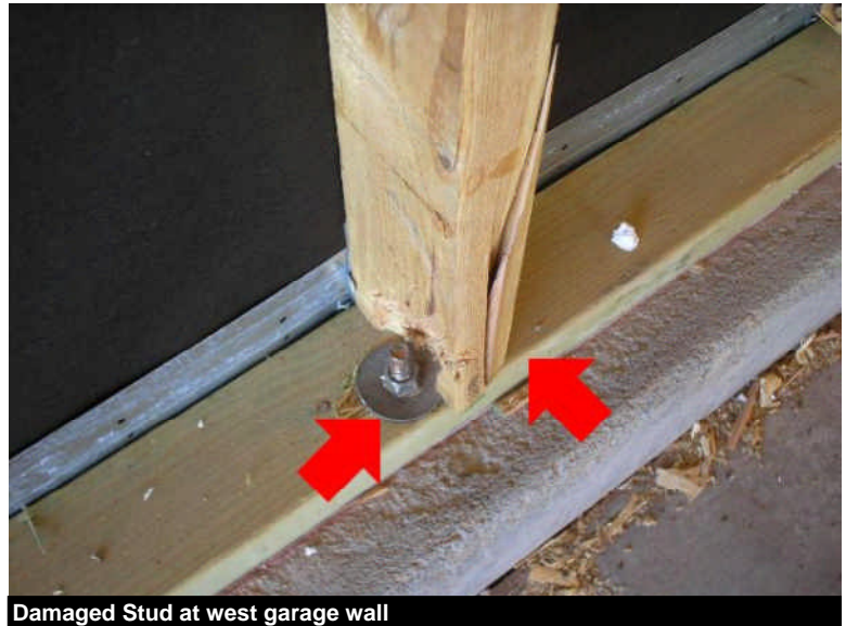
Damaged Stud at west garage wall
