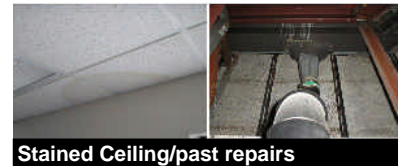
Stained Ceiling/past repairs
