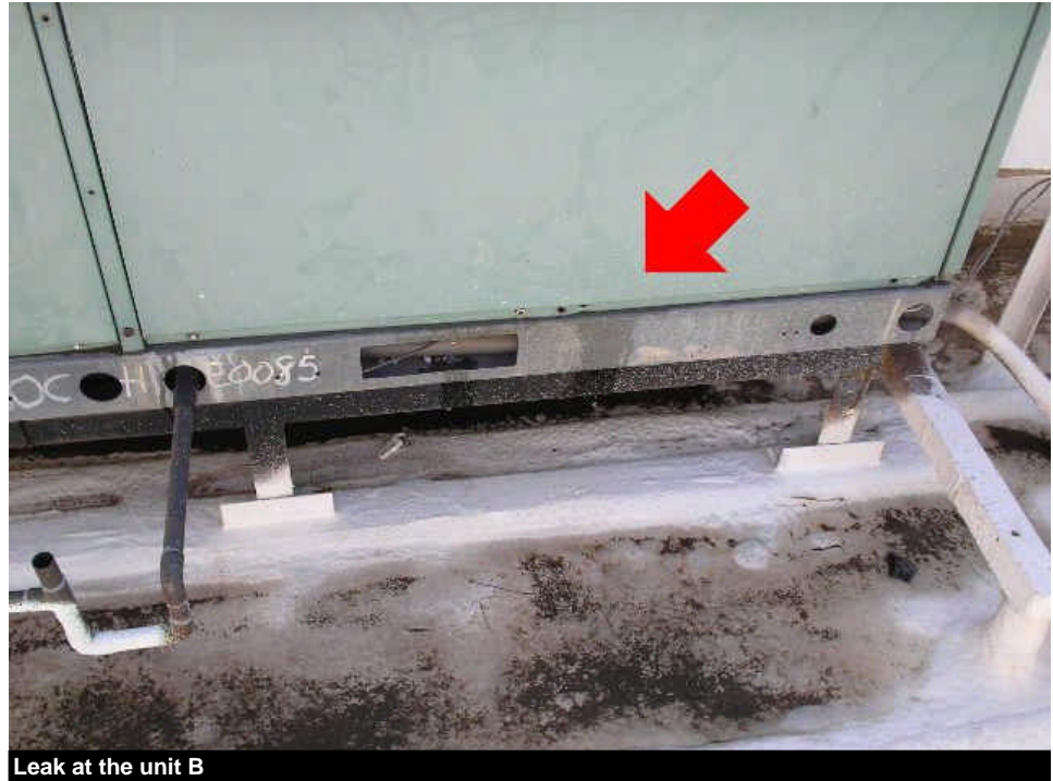
Leak at the unit B
