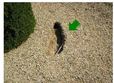
Holes at west side
