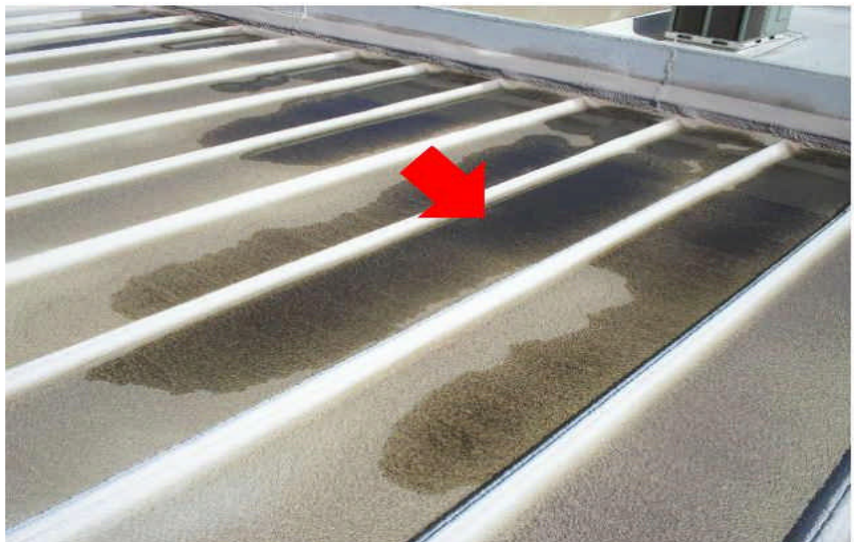
Water ponding and foam bubbles
