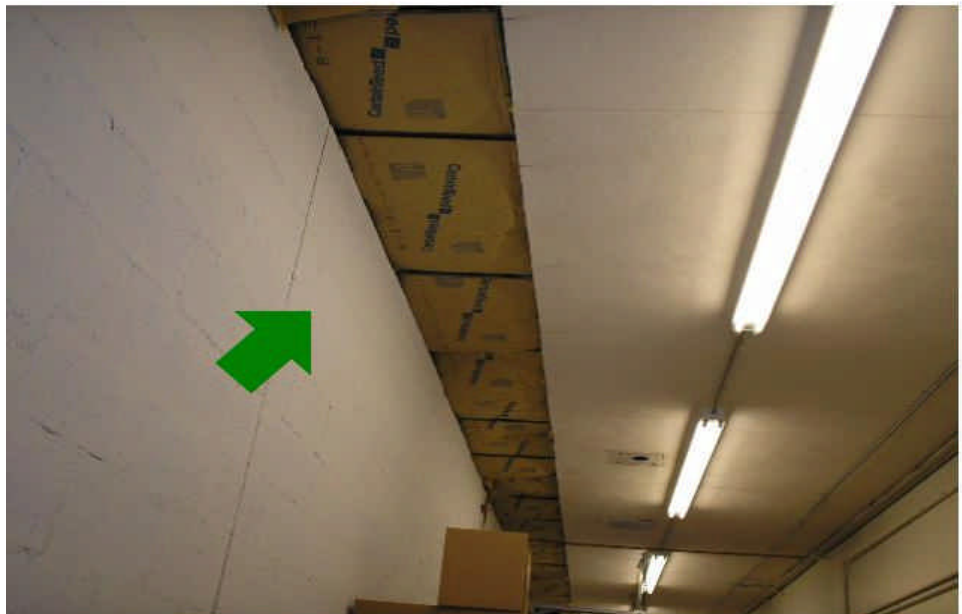
Misture stain and Missing ceiling panel
