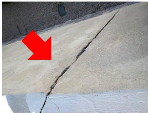
Cracks at masonry wall
