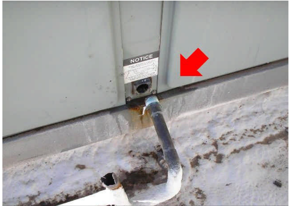
Loose condensate drain
