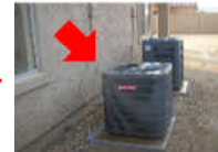
Missing insulation/4 units not level
